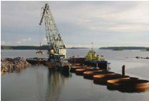
Fig. 1. Installation process of the basis for a transfer and elevation deck "Lukoil-II" from shells of major diameter (Vysotsk-city) 1
